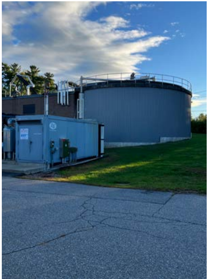
150kW co-generation system and anaerobic digester at the Waste Water Treatment Facility
