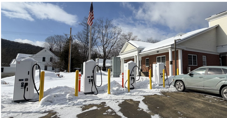
NEVI EV Charging Installation in Randolph, Vermont
