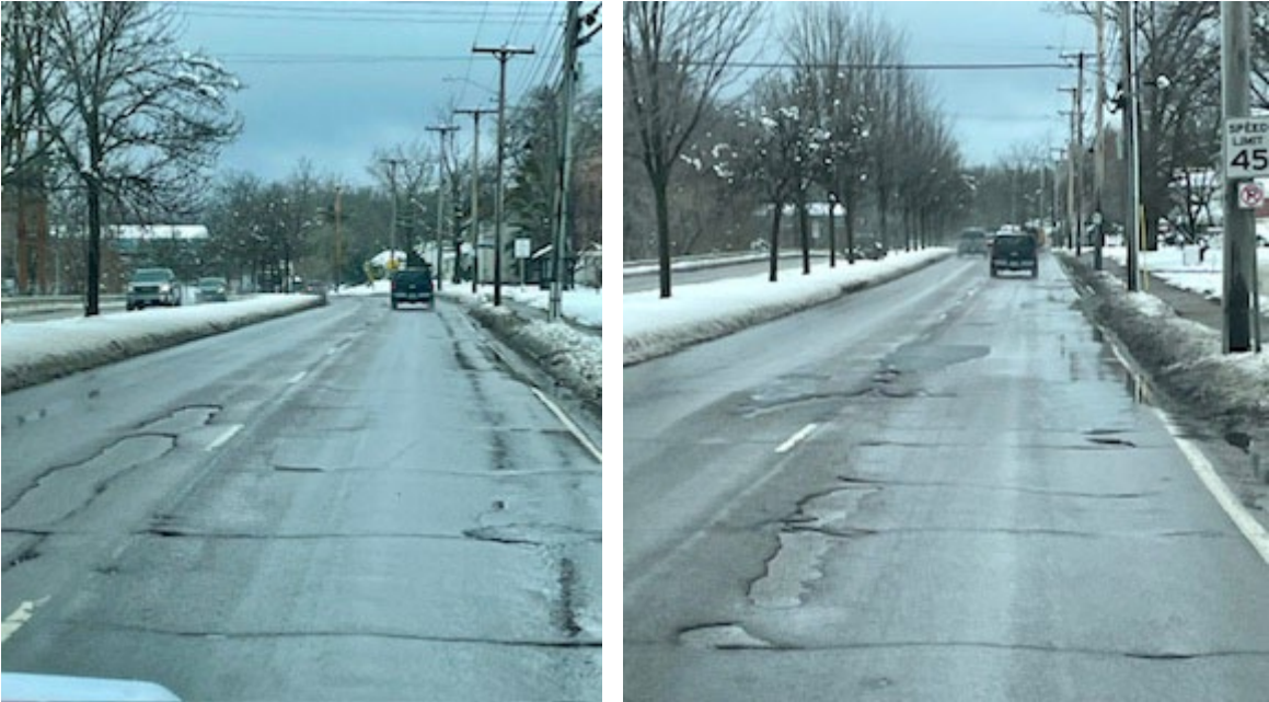
Figure 1: Conditions along Pearl Street (VT-15) between Susie Wilson Road and West Street Extensions as of April 2024. Based on Google Streetview, this segment was last paved in 2009.
