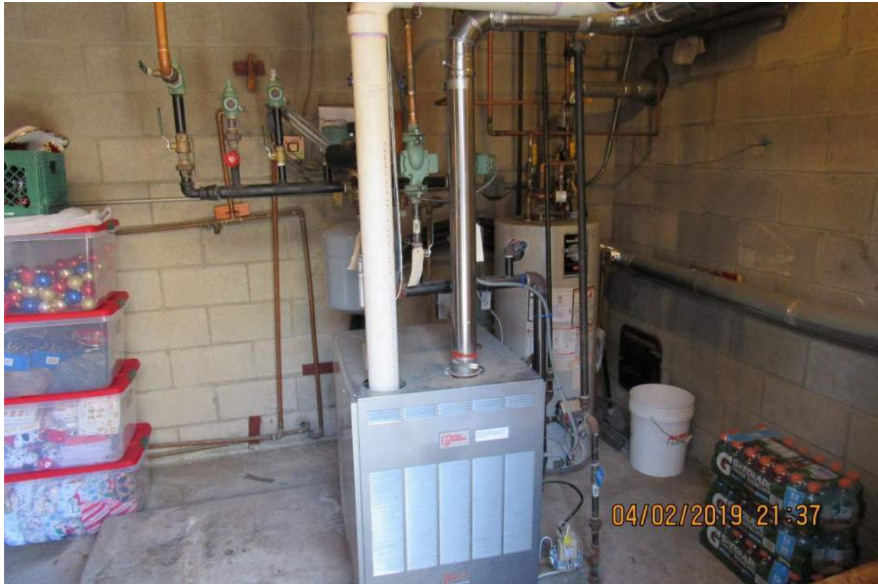
Boiler Room with Boiler; Note plastic storage boxes in Close Proximity
