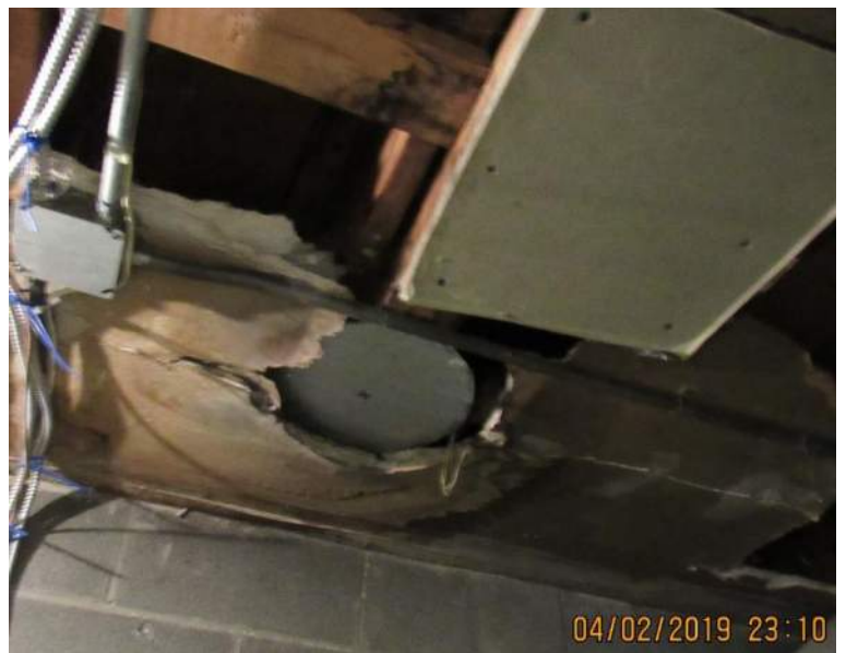
Failed Ceiling Boiler Room Floor
