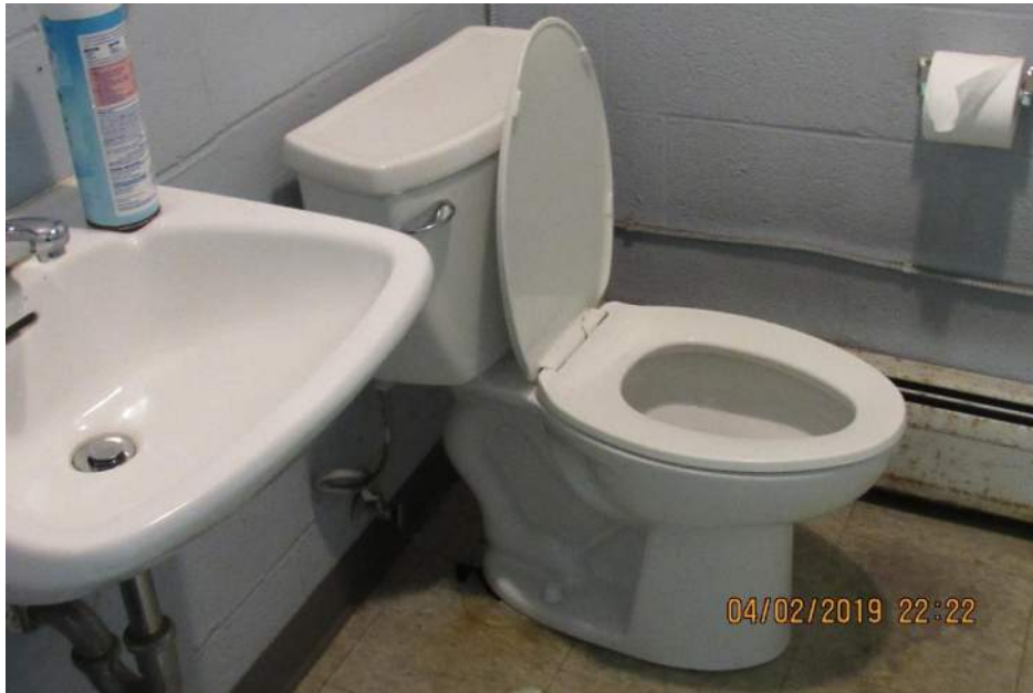
Sample Toilet Room; Note non-ADA hardware and rusted heating terminal unit.
