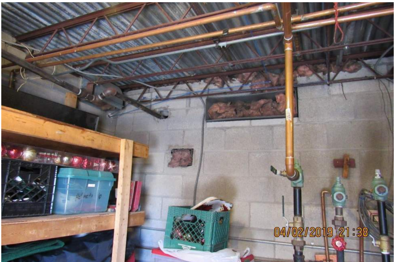
Boiler Room; Note Wall Penetrations and Wood Storage Racks in Close Proximity
