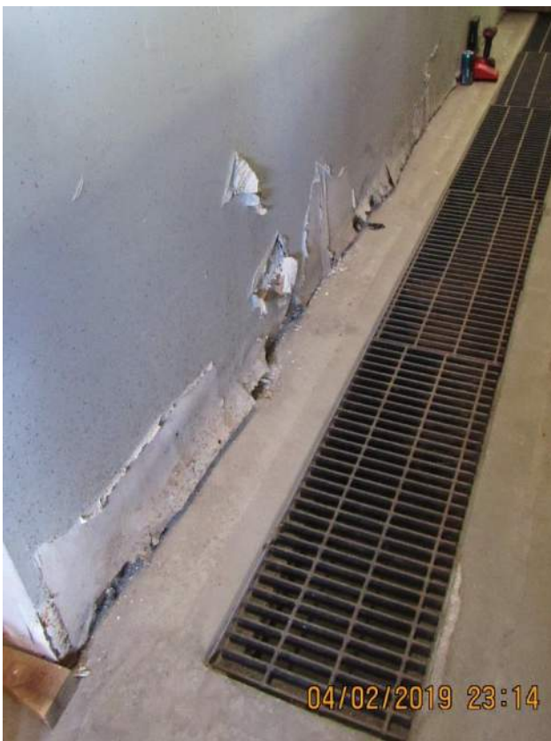
Apparatus Room Trench Drain with Water Damage on Wall.
