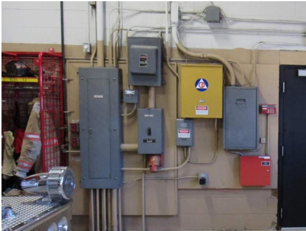
Older Electrical Panels and Disconnects
