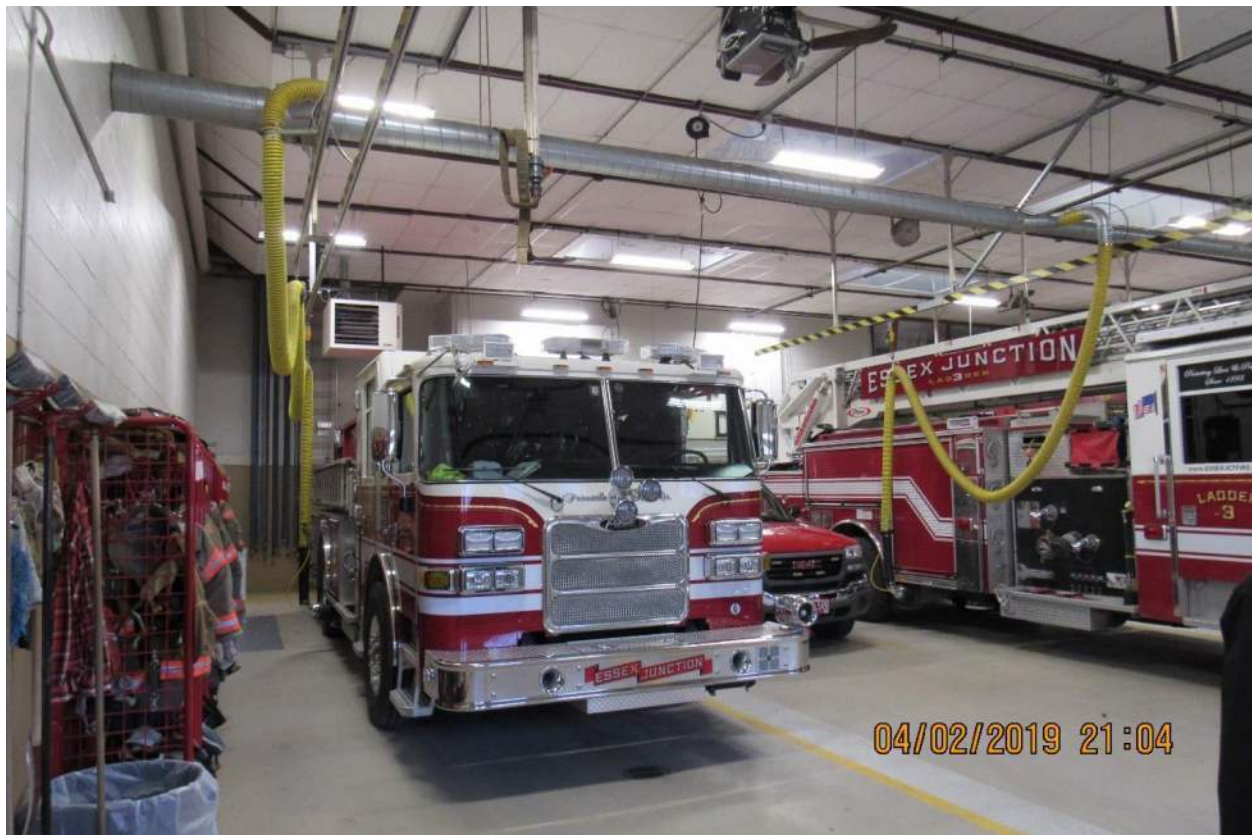
Apparatus Bay: Note Truck Exhaust and Electrical Drop to Vehicle. Tank Fill Hose is Wrapped on Ductwork (Not Used)
