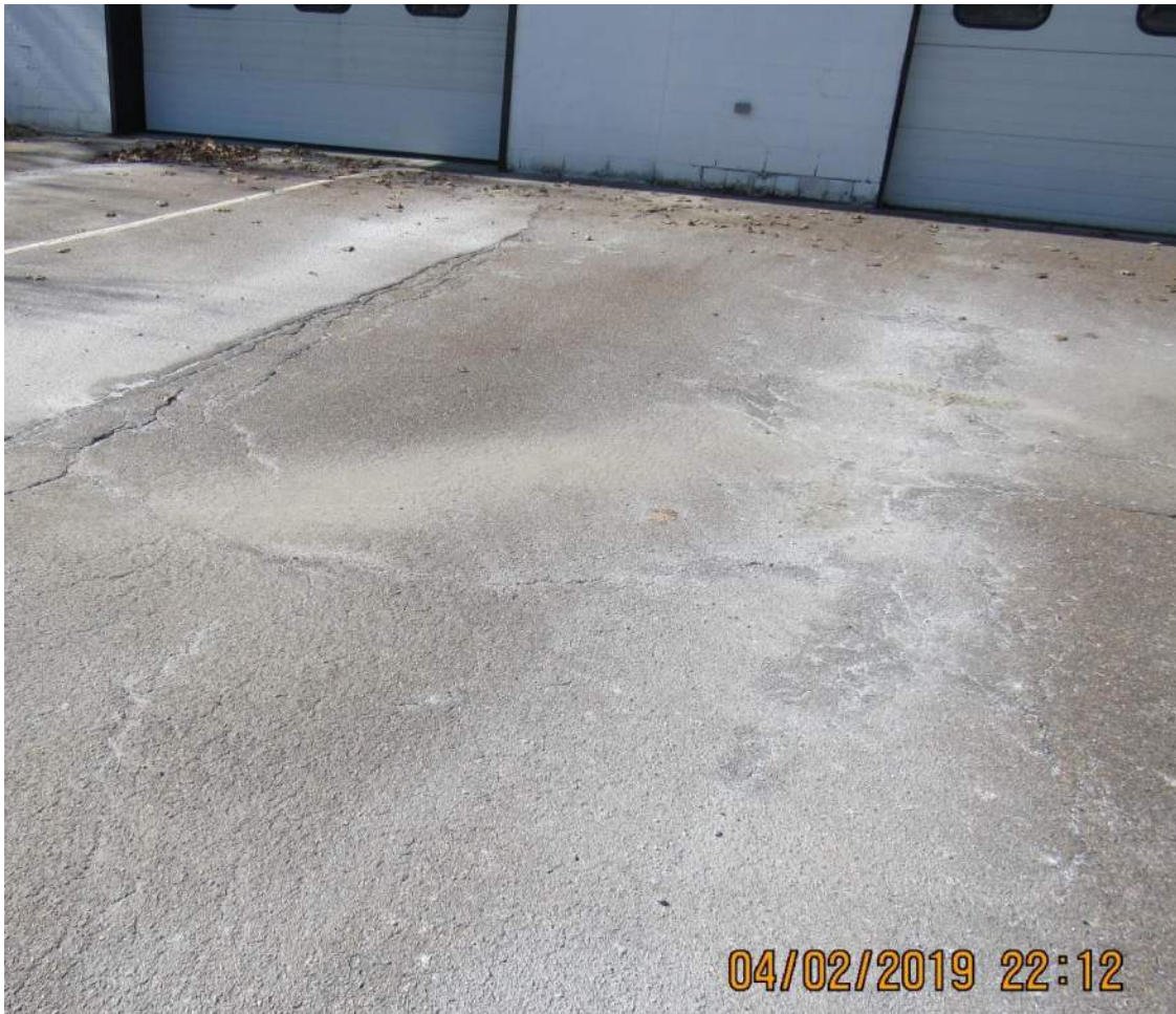
Supplemental Report Photo - Front Driveway: Note Damage Surface and Close Proximity of Masonry to Driveway Resulting in Evidence of Water Damage on the Masonry Wall.
