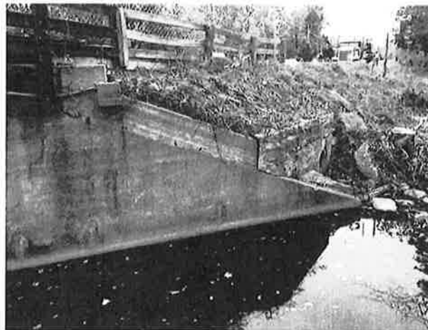
Photograph 1: Headwall Movement at Abutment No. 2
