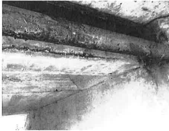
Photograph 3: Vehicular Bridge Spall Adjacent to Abutment No. 2
