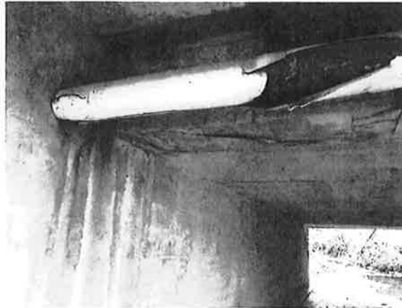
Photograph 4: Vehicular Bridge Spall Adjacent to Abutment No. 1
