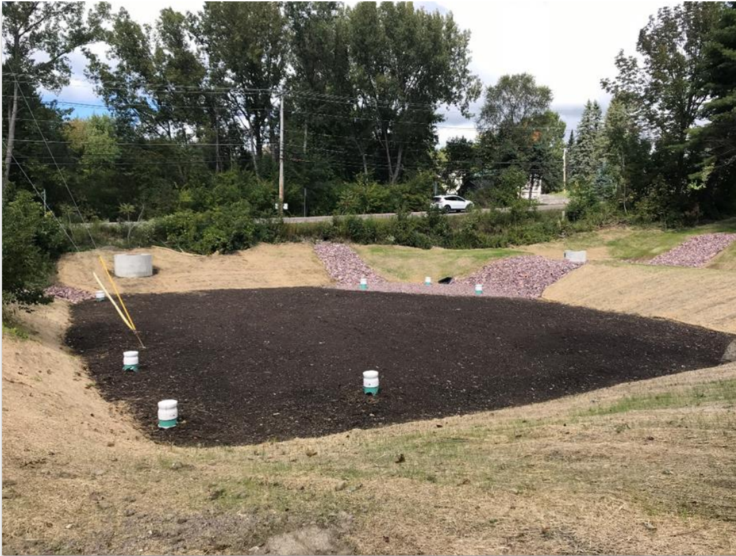
Completed construction of a stormwater constructed gravel wetland at the corner of Main St and Fairview Drive
