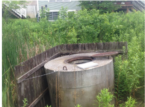
Figure 4: The Commons North Pond Outlet Structure
